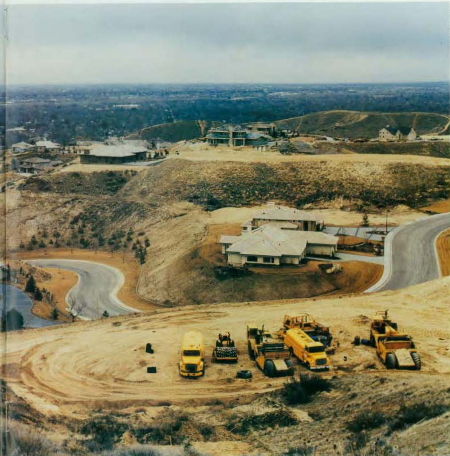
opers have been carving the Boise foothills into a series of terraces, leading to protests from downslope residents.
