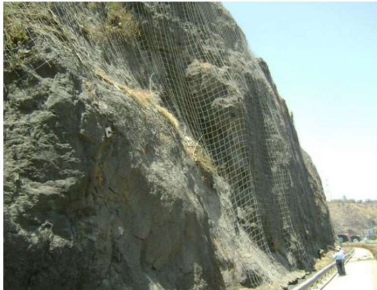
Figure 2.7: Cliff Face with Shotcrete and Steel Cable Net for Remediation
