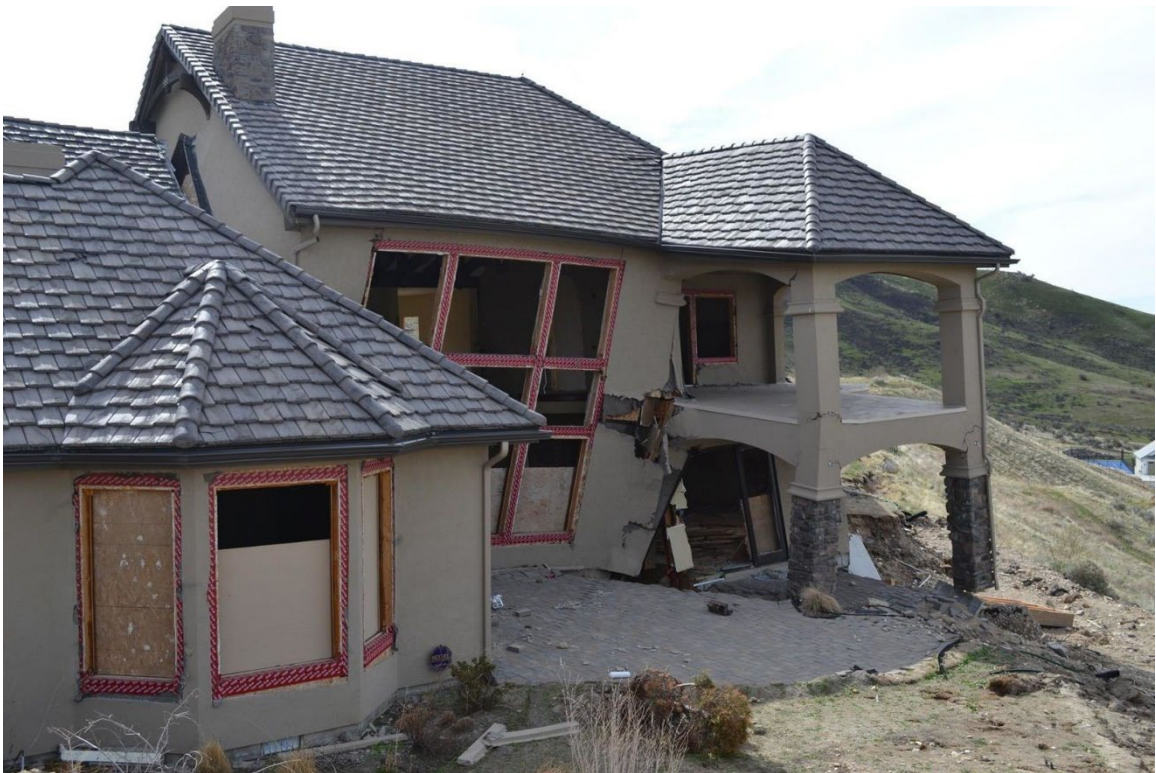
Picture 1. Damage at Alto Via Court
