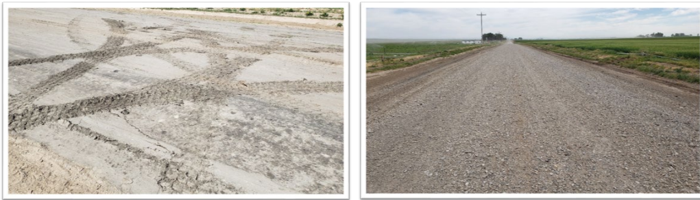
Pictures 3.1 (a) FIBP road base; (b) finished gravel surface upon project completion
