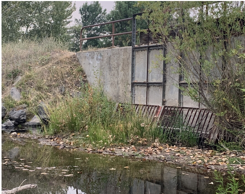
Figure 1.8 A closed irrigation gate on the Boise River. Courtesy T. Oppie
