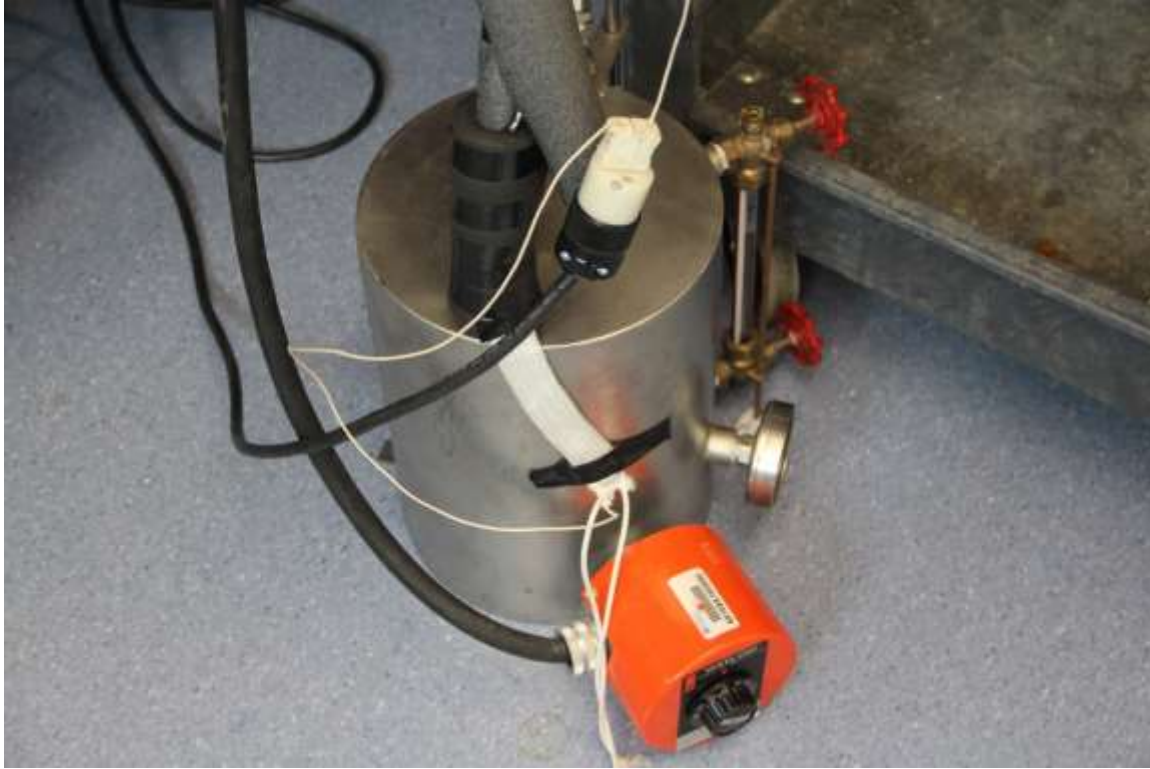
Figure 6.2 Environmental Chamber Boiler. This image shows the boiler used to generate humidity for the environmental chamber used in this test.
