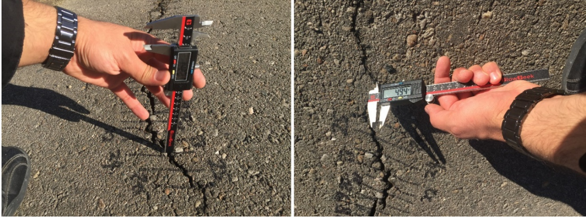
Figure 3- 6. Measuring depth and width of crack using digital caliper
