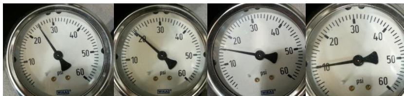
Figure 5.7 Sample Inlet Pressure Gauge Readings
