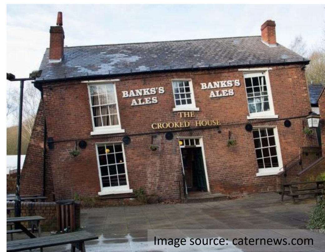
Differential settlement in foundation of a house built on expansive soil
