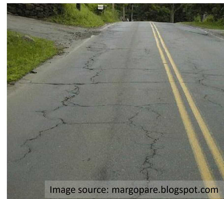
Cracks seen on a pavement surface built on expansive soil
