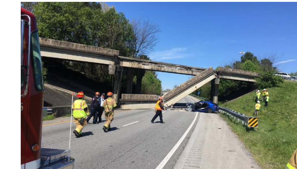
Bridge Collapse in Tennessee
