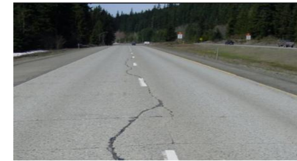
Pavement Damage due to ASR
