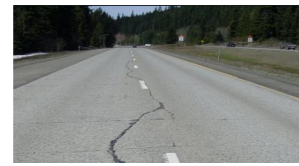
Pavement Damage due to ASR
