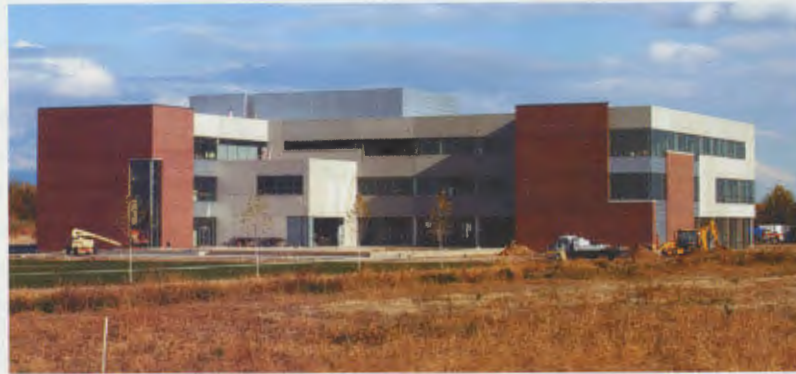
Construction of the academic building on Boise State's West campus in Nampa is expected to be completed by spring 2005.
