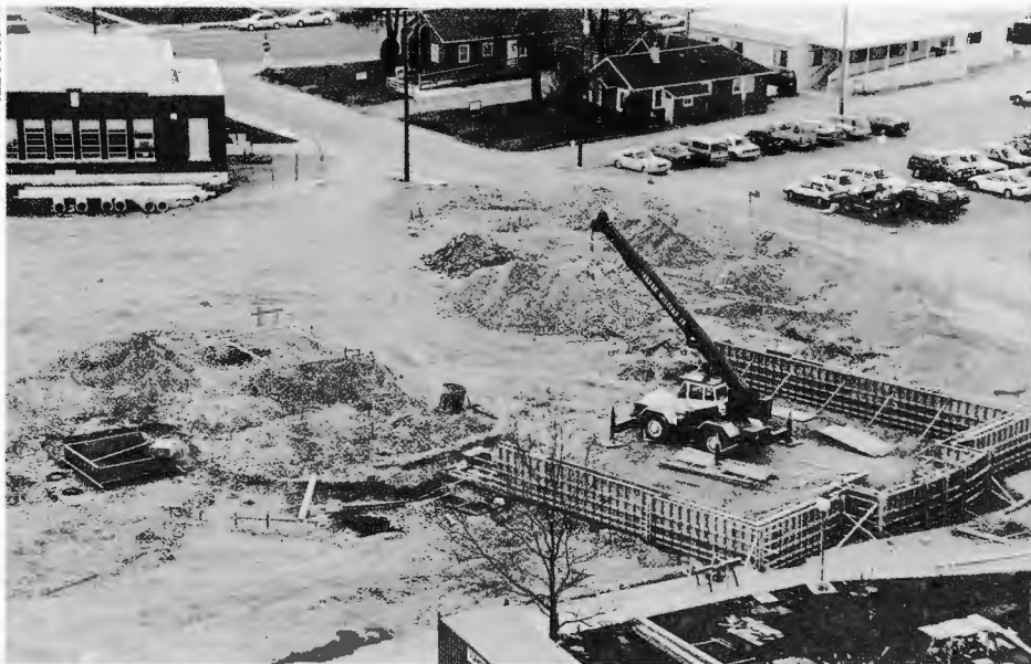
In one year the new multipurpose classroom building will rise from these foundations.
