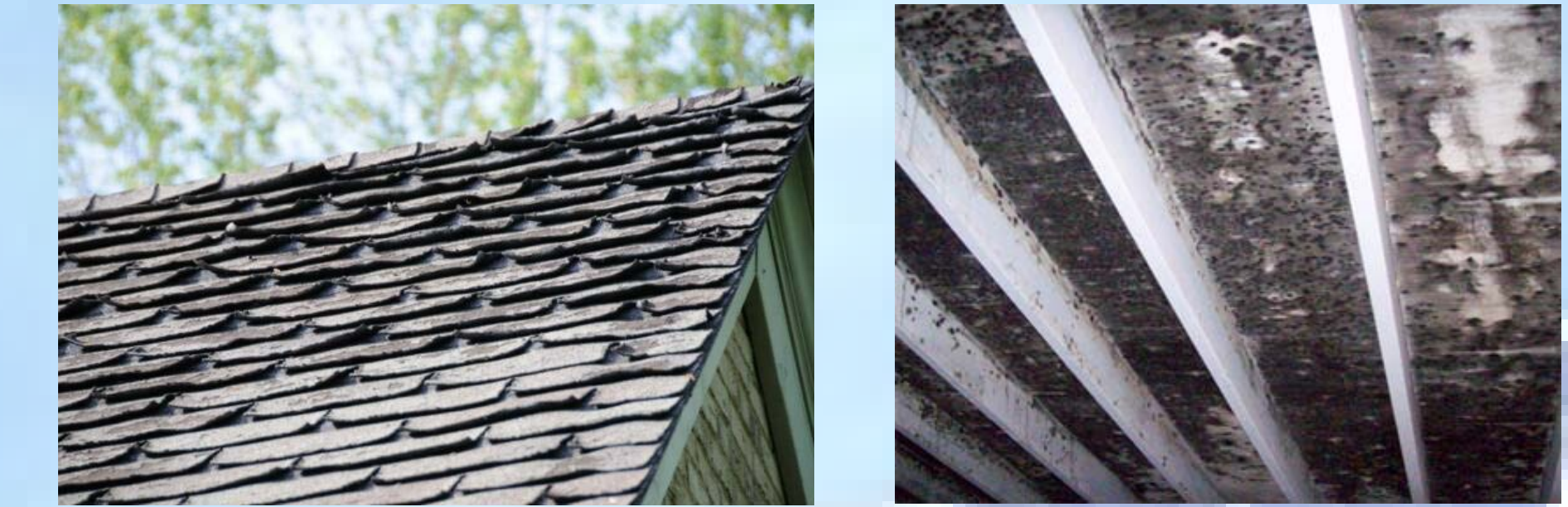
Curling shingles, and attic mold are results of poorly ventilated attic spaces.
