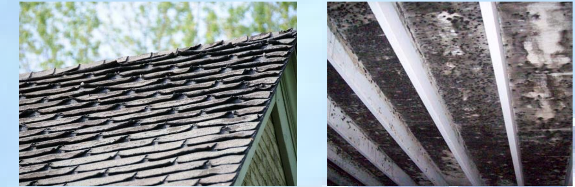
Curling shingles, and attic mold are results of poorly ventilated attic spaces.
