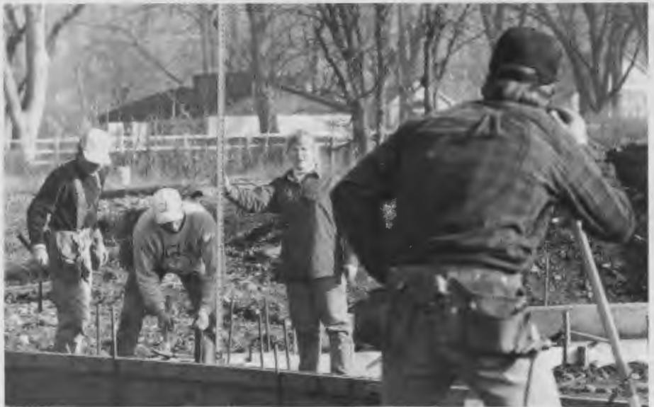
Members of the Award-winning BSU Construction Management Association helped with work on the Boise River Observatory, a 4.5-acre interpretive park near the Greenbelt.
